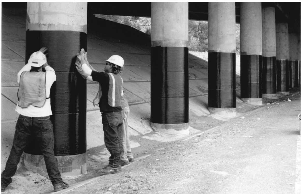
Figure 2.1b FRP wrap being installed on a highway column. (Courtesy of Sika Corporation)
