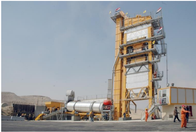
Figure 5.10 Kattameya Asphalt Mixing Plant (1)
