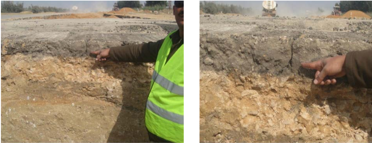
Figure (3.3) Cracks extended to base layer
