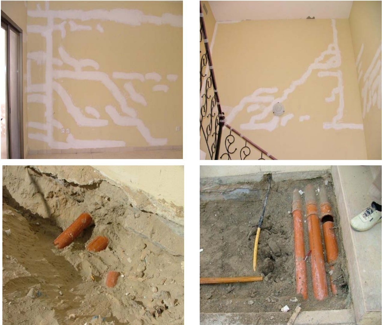
Figure (3.9). Gardens Hillside View Villas cracks, and broken sewerage pipes due to the differential settlement
