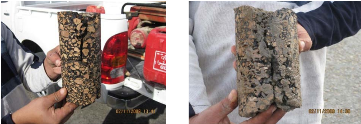
Figure (3.4) Core sample on cracks shows deep cracks along sample
