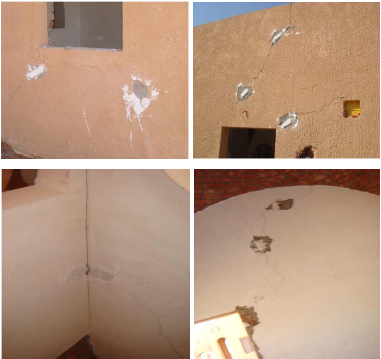
Figure (3.7) Factory buildings cracks
