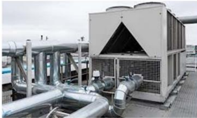
Central air conditioning (chiller)
