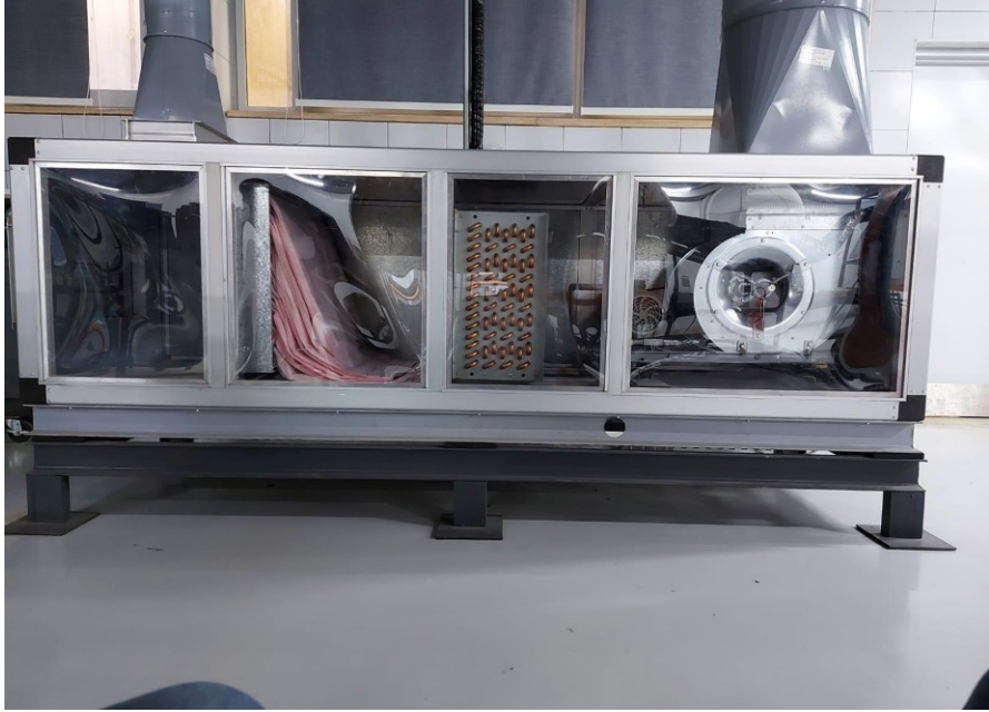
Figure 1.33 Air Handling unit full scale unit
