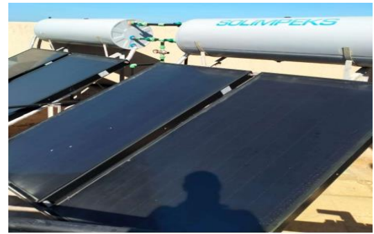
Figure 3. Installed Solar Heaters
