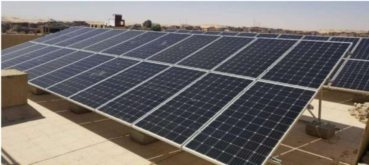
Figure 2. 150kW solar power station in Aswan campus
